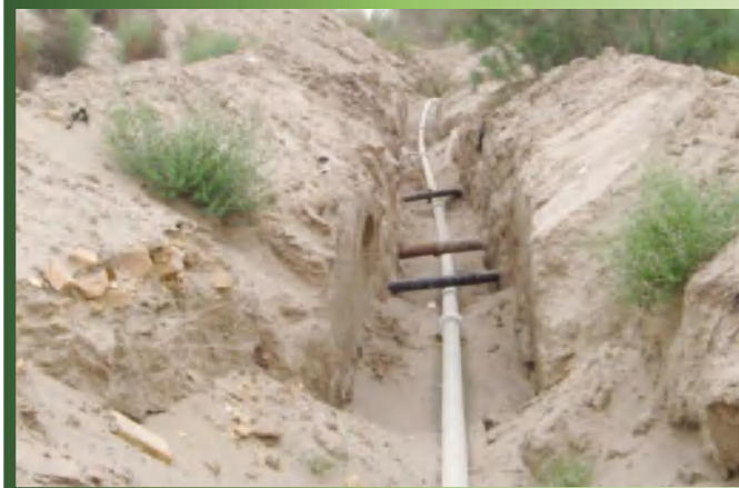
DN80mm PN25MPa GRE Pipeline Project for Injecting Water Injection to Carboniferous Block 3 of Northwest Oilfield, Sinopec Specification: DN80mm, PN25MPa
