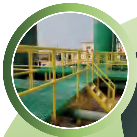
Protruded platform and grating for chemical plants
