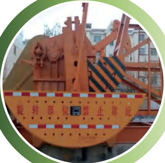
Protective cover for pumping unit Wellhead guard
